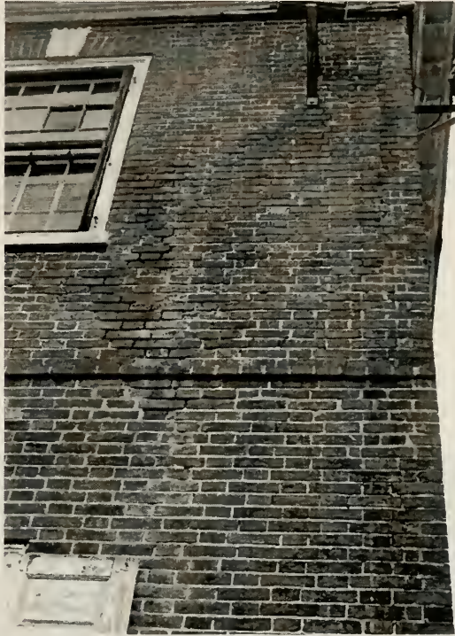
Figure 24 Brick Saturation Through Capillary Rise, Efflorescence and Mortar Erosion, 1998 Photograph by Author
